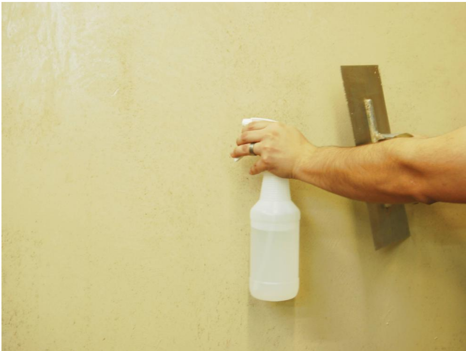
Lightly mist the Tierra™ with water and trowel down to compress and smooth out.
